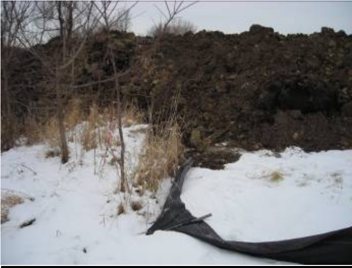
Wetland and upland spoil not separated at DA-W5 boundary Report 4-DD-094 – 1/16/08
