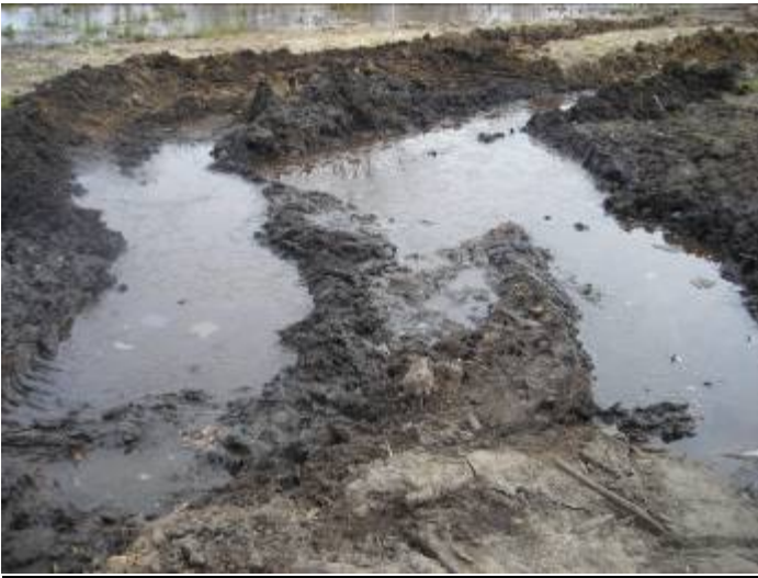
Location where track hoe walked off the mats in Wetland Report 4-DD-076 – 11/10/07
