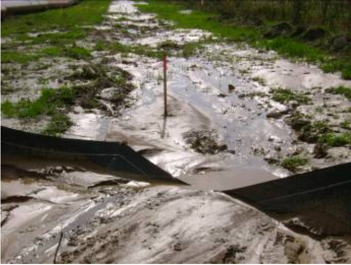
North end wetland RU-W83. Sediment entering wetland where silt fence is in need of repair. Report 2-JV-116 – 10/6/07
