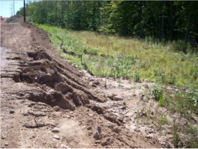
Sediment, ECD Blowout in wetland Report 1C-ST-020 – 8/30/07
